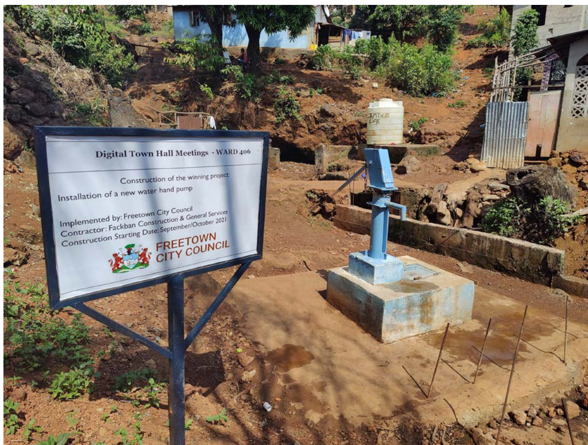
FIGURE A5. Hand Pump Implemented in Ward 406
